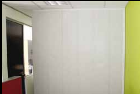
▲ Install full height or free standing walls to any size/shape.
